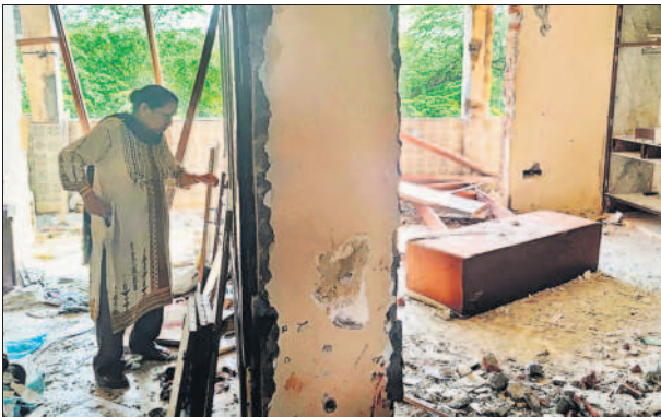
Between 30 and 50 flats were still occupied at Signature View Apartments when utilities were snapped. VIPIN KUMAR/HT PHOTO
